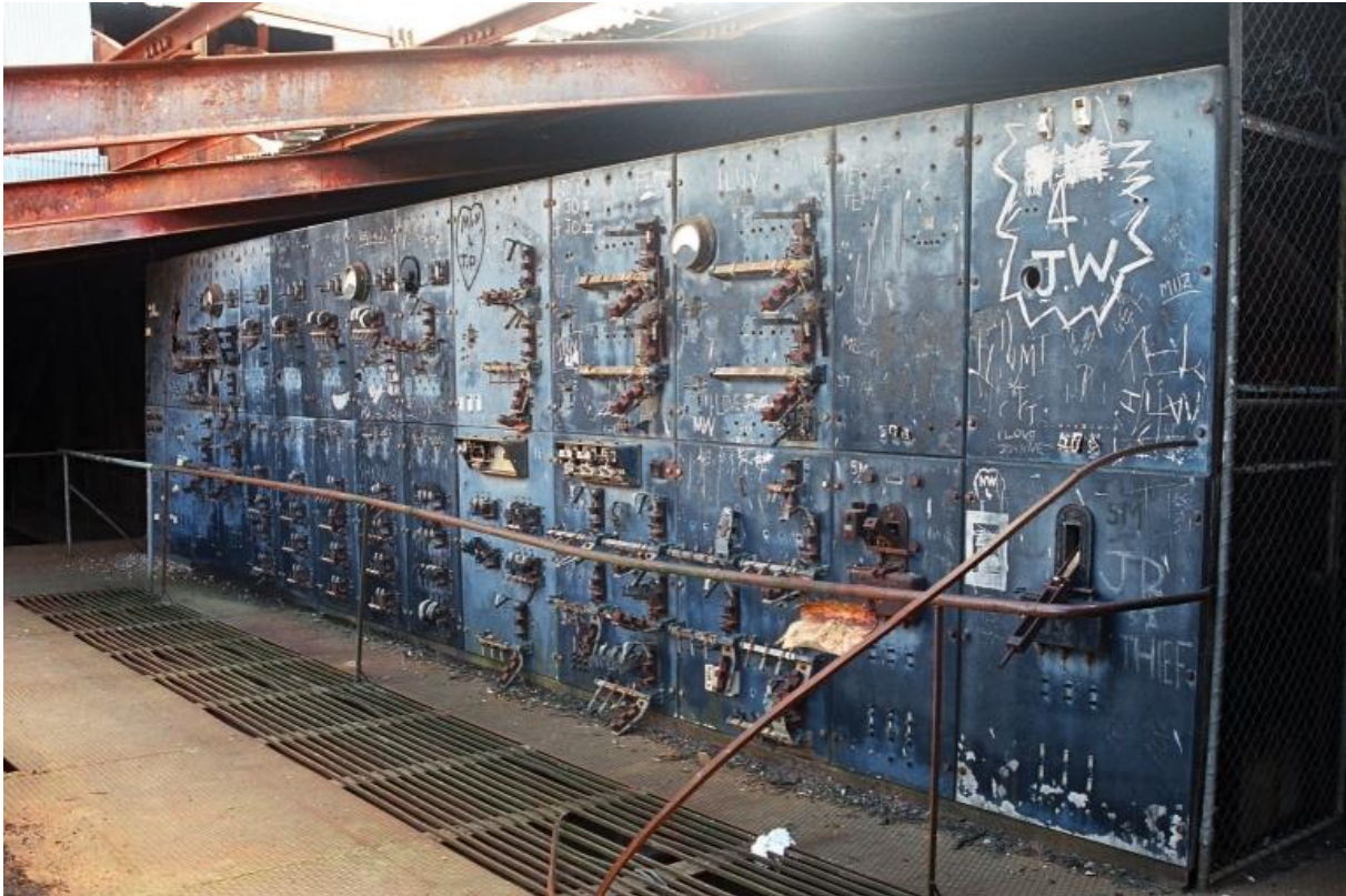
Figure 15: Switchboard in the Control Room as seen in 1994 with electric meters and manual switches (some open blade type) that monitored and controlled the various motors. Since then all meters have been smashed and some copper components and wiring stolen. Note the sparse safety guardrail. The grid floor panels gave the Winchman a view to the winches below. The cgi roof cladding above the Control Room was stolen, but has since been replaced. (Photo by C. Doring)
