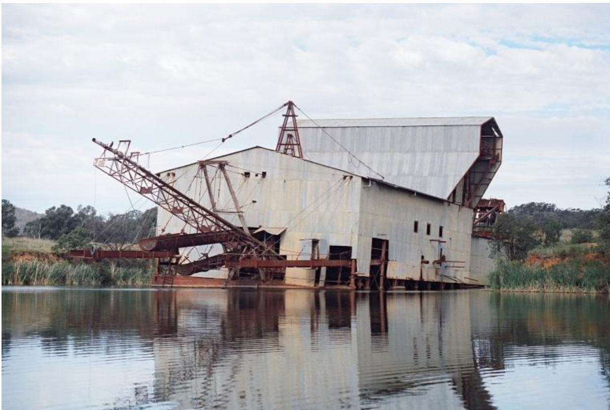
Figure 4: Stern view of the dredge, seen from SW. Note the tilt towards the front-right corner. Note also how the upper part of the tall central superstructure protrudes to allow the manual overhead crane to move heavy equipment on or off a barge alongside. (Photo by C. Doring 1994.)
