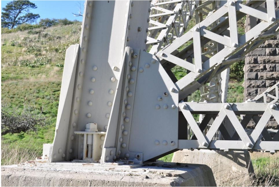
Moorabool Viaduct, 2010. Fabrication details of one leg of one of the trestles - Dorman, Long & Co. Ltd. c1918.
