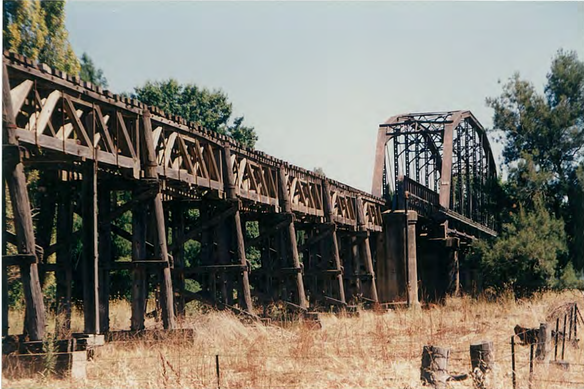
The railway timber viaduct and the steel truss over the Murrumbidgee River. The maker's plate is attached to the end steel post on the right hand side.
