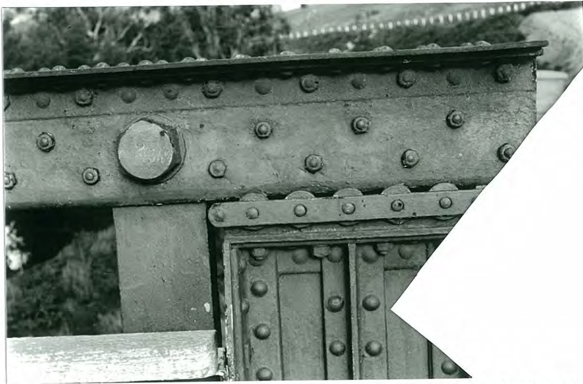
The unusual bearing arrangement on the Prince Alfred Bridge. Here at the end of the bridge, the cantilever stub of the top member sits on a linked set of 5 rollers which sit on the riveted vertical post which rests on the tops the piers, below. On the left is one of a vertical members of the truss which restricts the amount of movement of the rollers. A similar arrangement supports the continuous top member over the inner piers.
