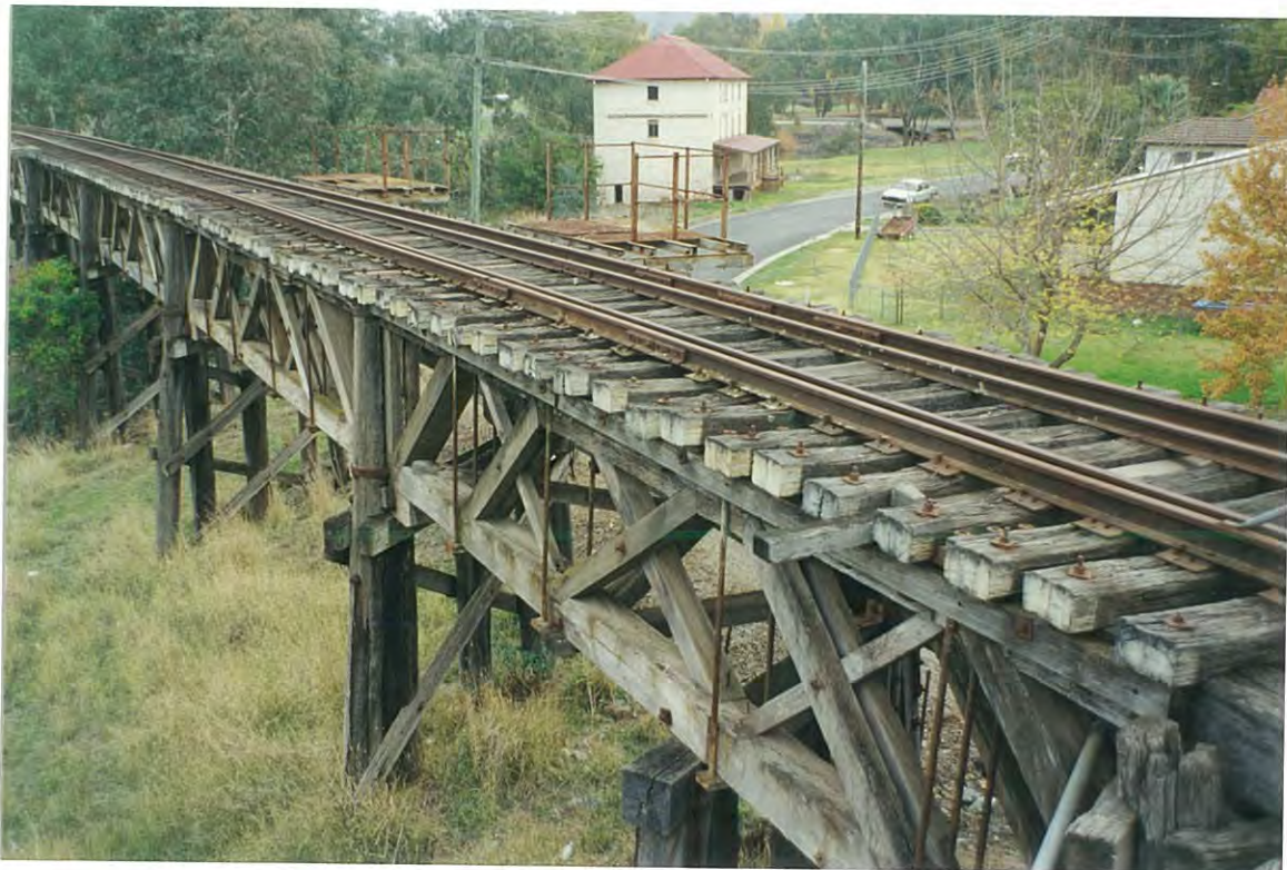
The timber truss railway viaduct at the Gundagai end. As a cost saving measure the timber joints at the ends of the members are shaped or scarfed so as to fit together thereby transferring the structural forces. On timber truss road bridges these joints incorporated expensive cast iron plates to ensure a good fit.
