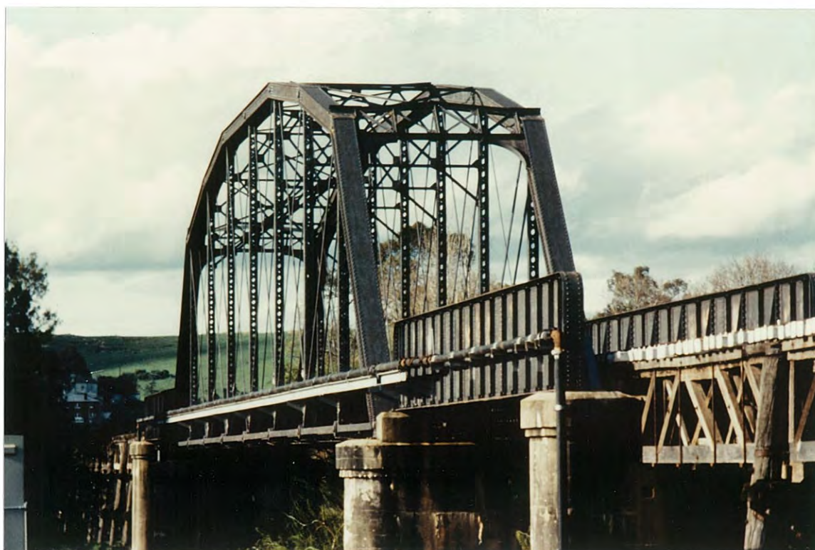
The hog-back style of the Gundagai railway truss flanked by its plate web girders. The pins can be more clearly seen in the top chord but are also in the bottom horizontal member.
