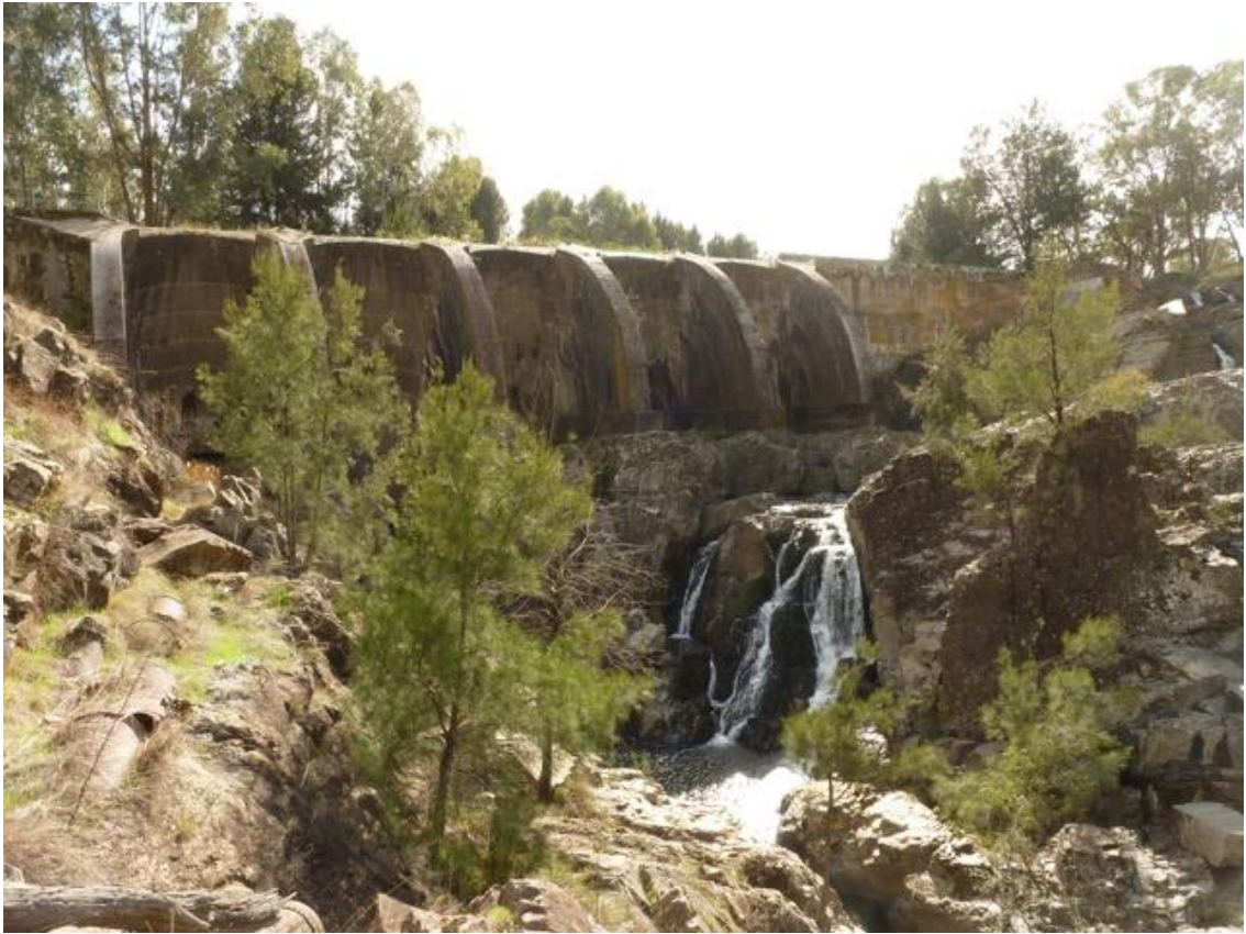
Junction Reefs Dam from downstream, early 2016. Note remnants of penstock at left. Image: Miles Pierce
