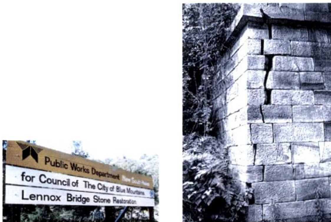
Figure 6 Restoration acknowledgements and typical damage to stonework of Lennox's Horseshoe Bridge (Henry Kullas and DPW&S).
