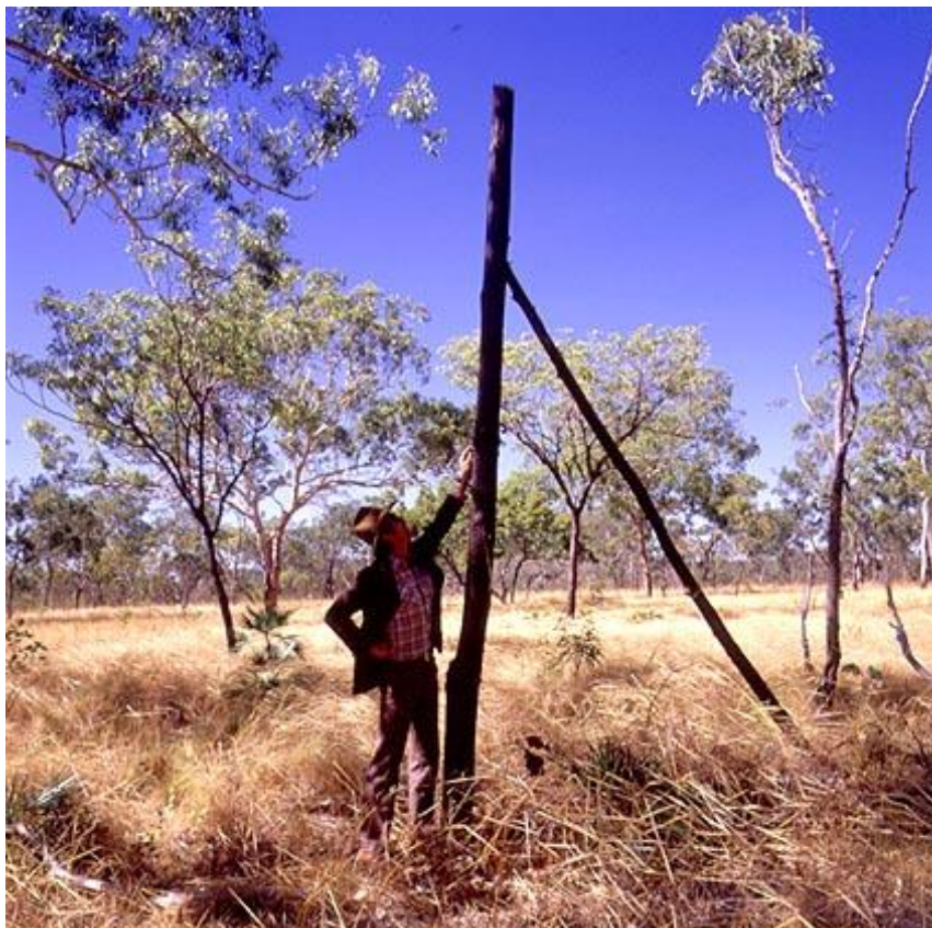
Typical original timber pole. This is an angle pole with a compression brace still intact, located north of Pine Creek. Image taken in 1984.
