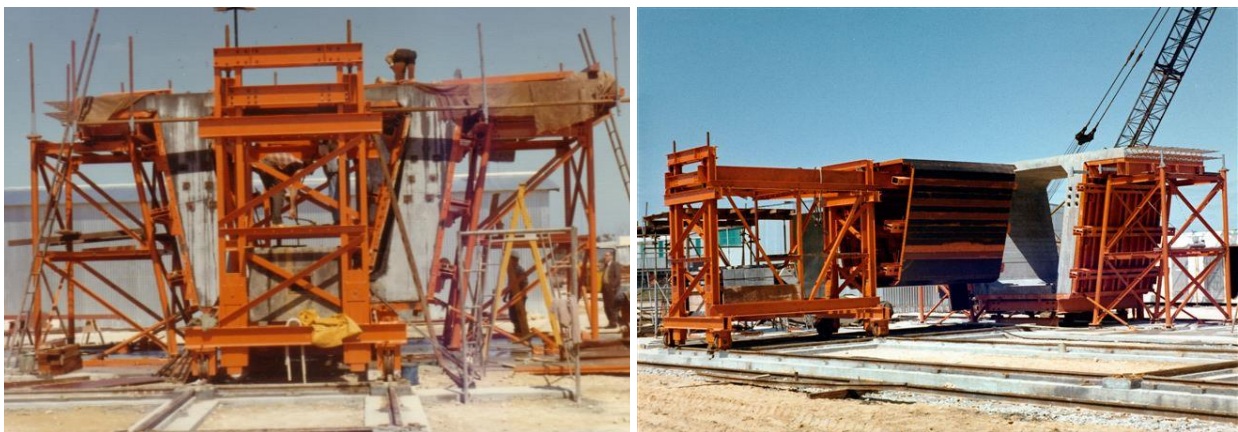
Figure 6. Precast beam unit travelling steel forms - internal form being released (Photos J O Clough & Son)
