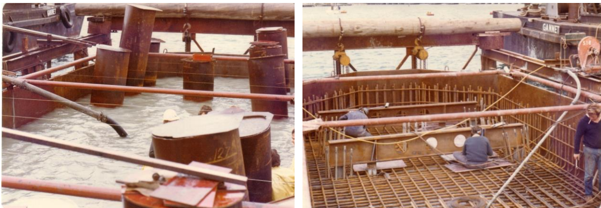
Figure 7. Left: Dewatering the pile cap; Right: Placing the hanger beams to transfer pile cap loads to the steel piles (Photos J O Clough & Son)
