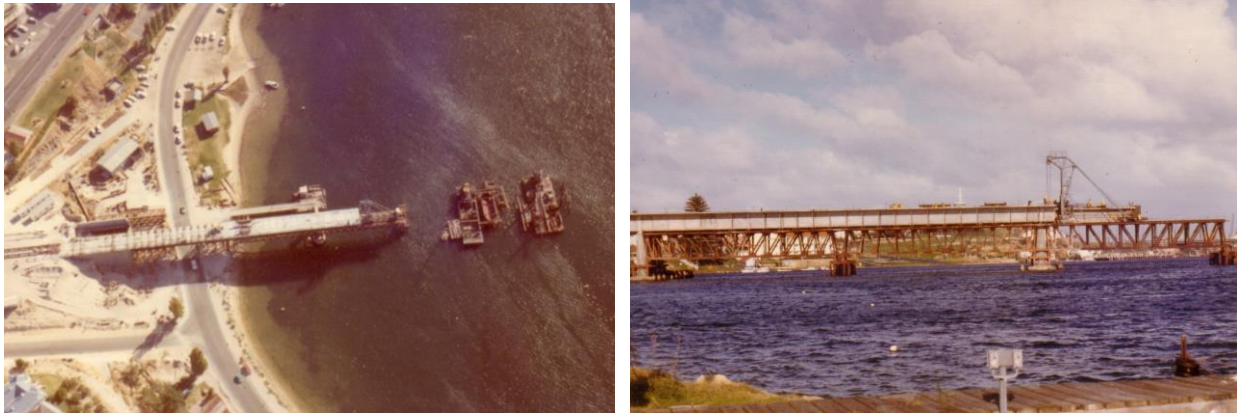
Figure 13. Left: Progress near completion of Stage 1, Feb 1973; Right: Progress near completion of Stage 2 (Photos J O Clough & Son)
