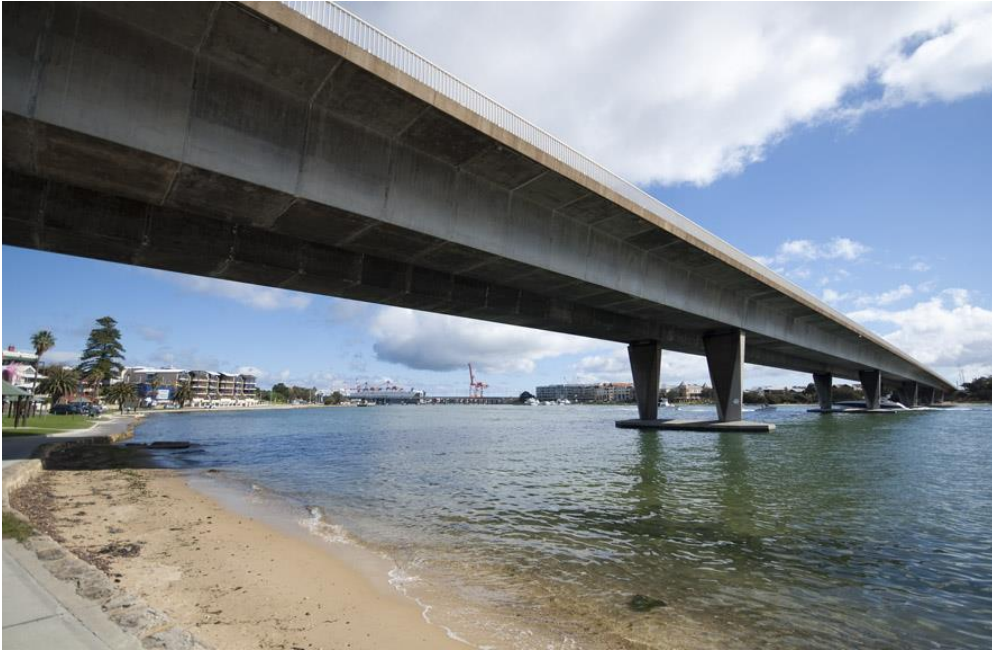
Figure 4. View of the Stirling Bridge looking west towards the port of Fremantle (Photo Anthony Riddette)
