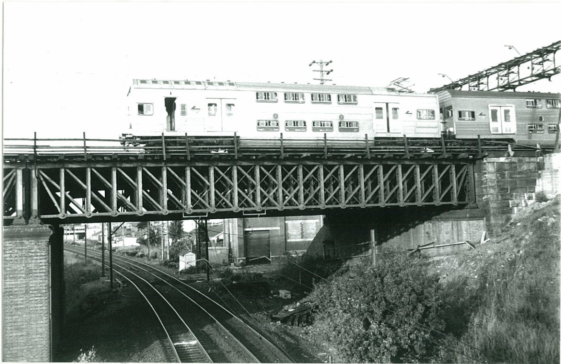
One of the three sets of Whipple trusses at Lewisham prior to replacement.
