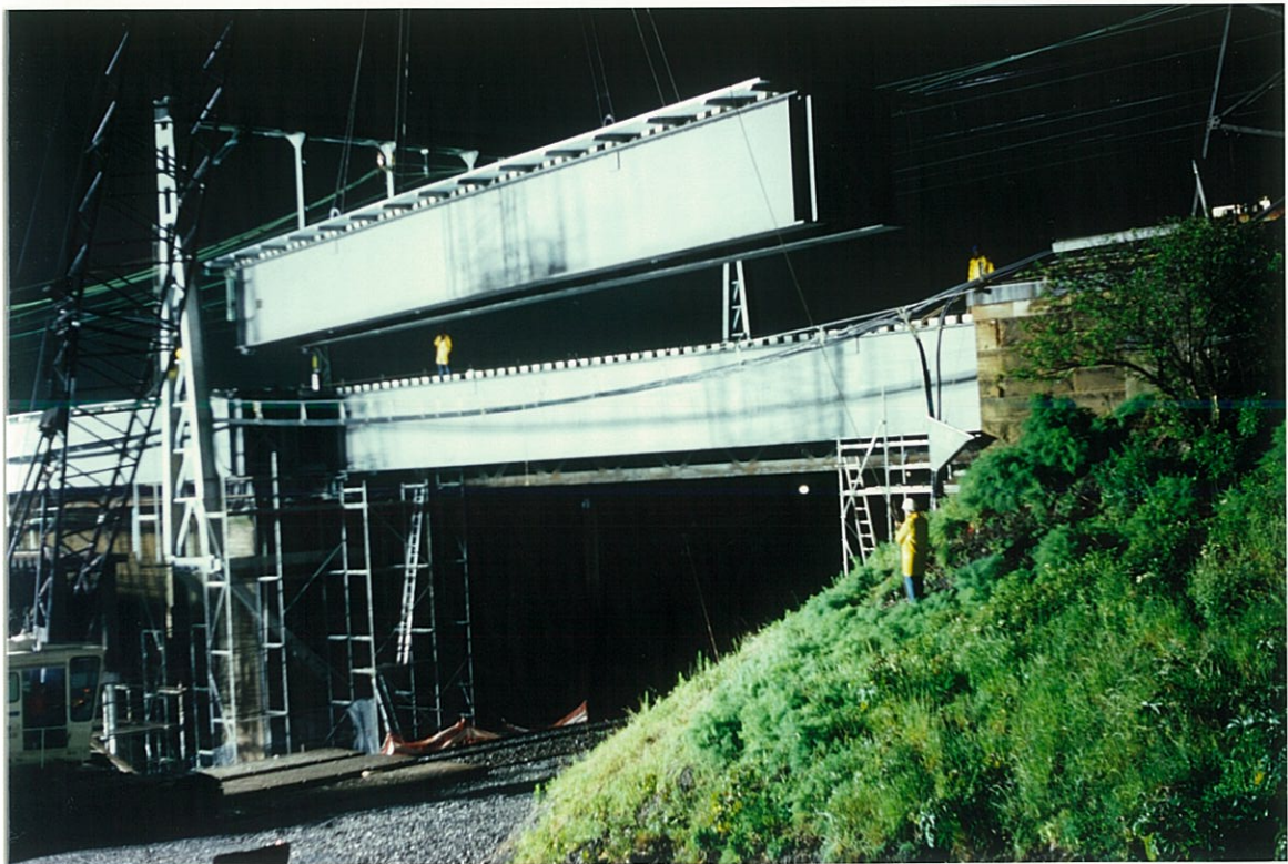
The last plate web girder about to be positioned 11pm 3rd October, 1993.
