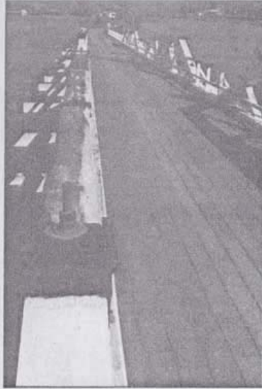
Figure 2.3.2f – View of truss showing single rods all of which are the same size
