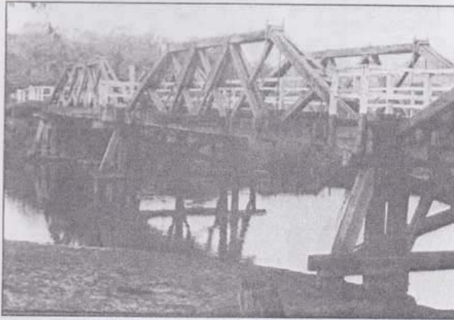
Figure 2.3.3a – McDonald Truss - Junction Bridge at Tumut remains in use to this day.
