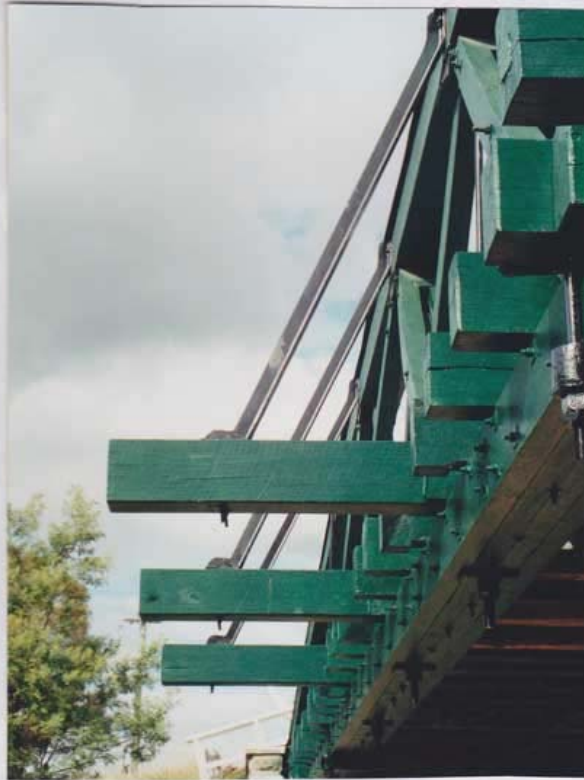
McKane's Bridge, opposed metal wedges are at every bottom chord joint to take up the timber shrinkage. They are a significant feature of the McDonald timber truss. Below, a set of rakers supporting the top compression chord against lateral buckling.
