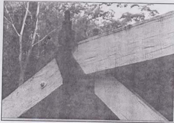
Figure 2.3.3d – Vertical rods placed outside the truss faces eliminated the need to drill through the top chord.
