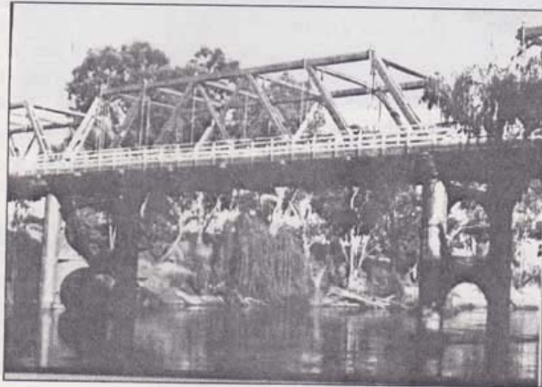
Figure 2.3.4e – Hampden Bridge, Wagga Wagga. The first of Allan's large overhead through truss bridges with 3 truss spans, each of 110ft (33.5m).
