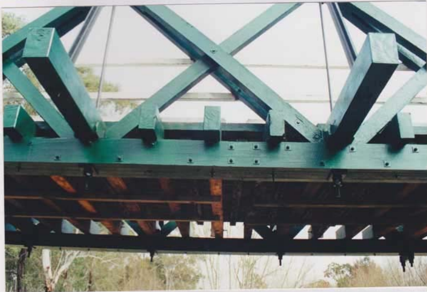
McKanes Bridge, the short thrust block between the ends of the sloping end timbers of a McDonald timber truss. Bolts connect this to the longer bottom chord in tension. Below, closely spaced cross girders resting on the bottom chord between the main joints, add bending to the bottom chord.
