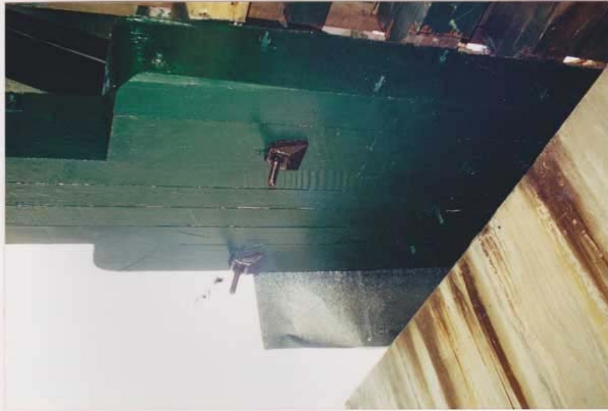
McKanes Bridge, the underside of the deck system, longitudinal planks on closely spaced cross girders and bolting strips. Below, the bottom chord made from 4 parallel flitches plus widening at the pier support.
