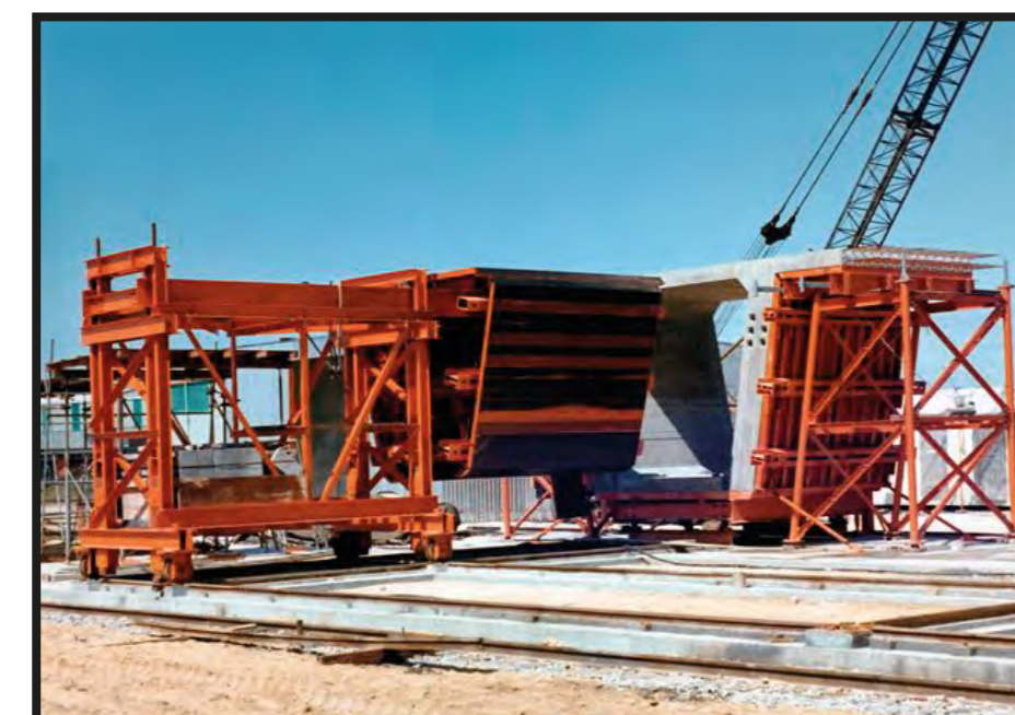
Each concrete beam unit is slightly different. Adjustable forms were used to ensure all 292 units were accurately cast
