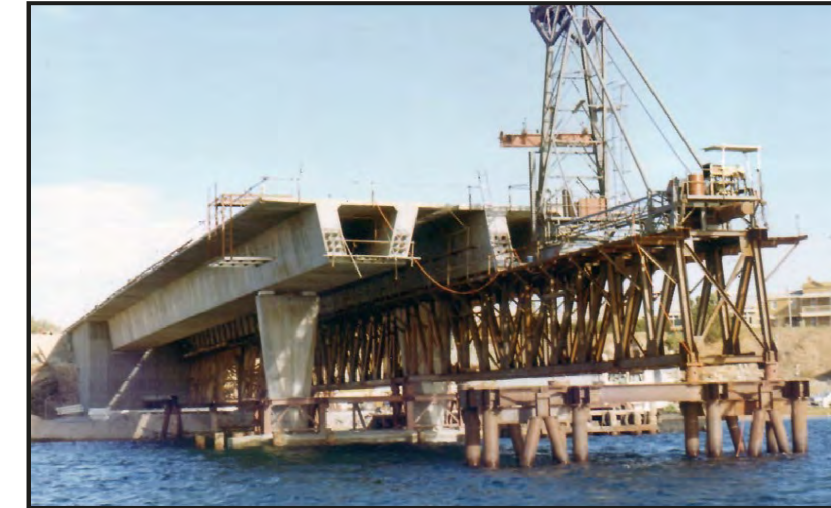
Stage 1 construction, showing completed upstream row and temporary piers supporting the falsework truss and placing gantry. The downstream row is nearing completion.
