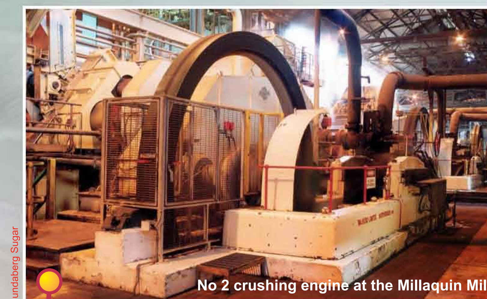
No 2 crushing engine at the Millaquin Mill
